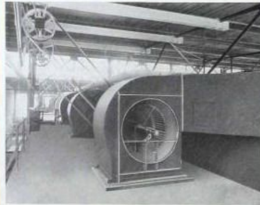
H. W. Johns-Manville Co., Manville, N. J. Battery of "Sirocco" Fans for dryers, Factory has complete "A B C" Equipment.
